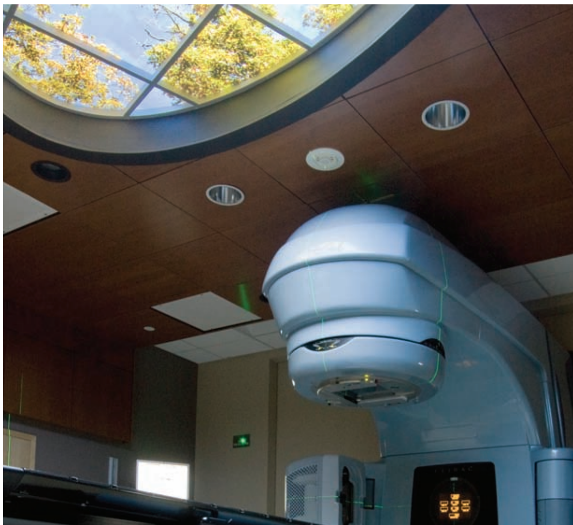
Radiation vaults provide radiation therapy for lung, breast, prostate and colorectal cancers.
